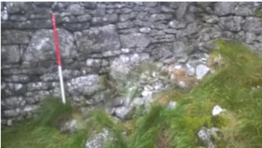
Pile of fallen stones against west gable prior to removing grass sods.
