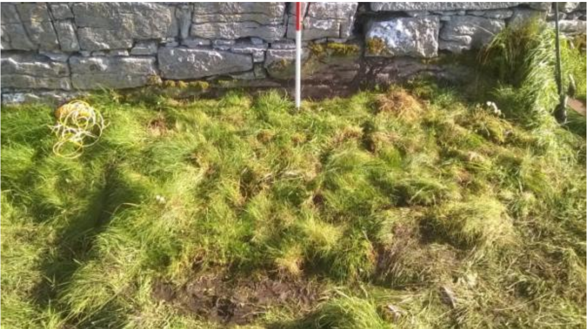
Site backfilled and re-sodded. 1-9-2017 Stain on wall shows the height of the excavation.
