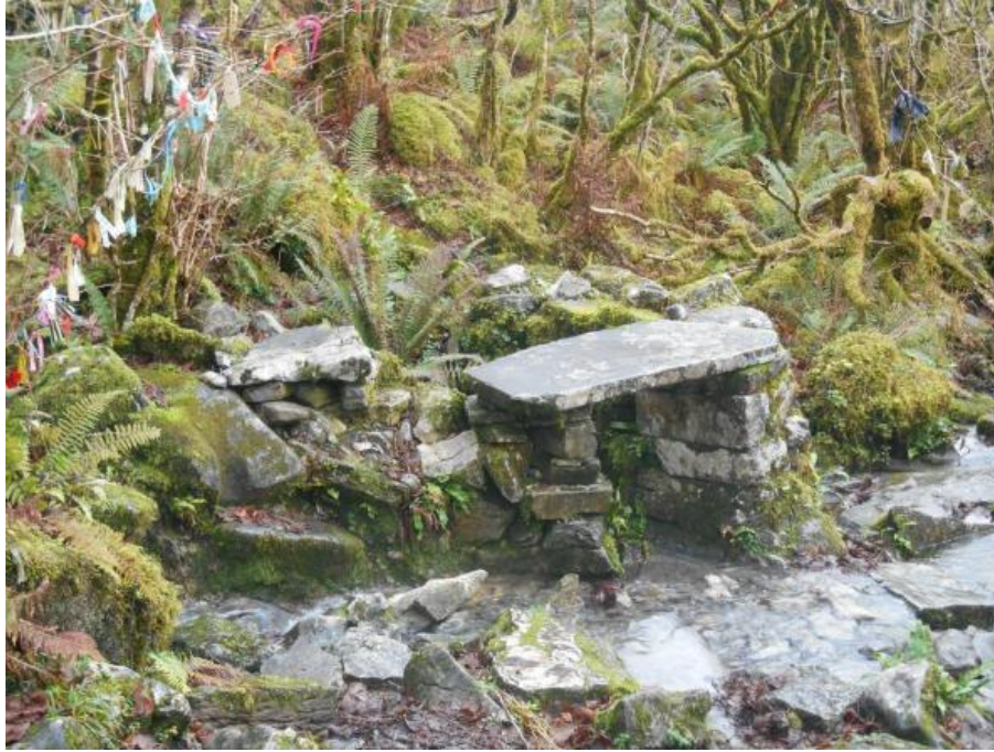
Photo 9. Partial collapse of well house. Left of lintel/slab.
