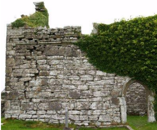
Photo 8: Ivy growth over south doorway and cracks in wall 2005
