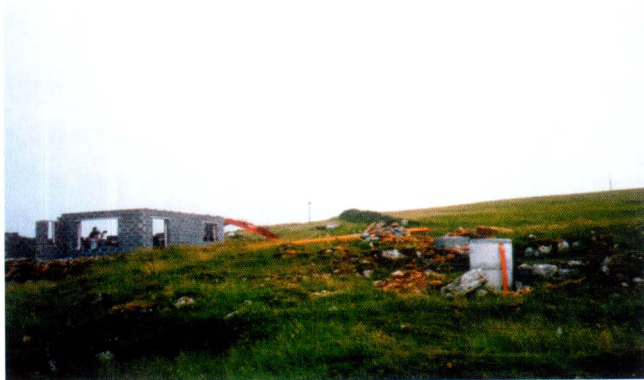
Construction of a bungalow and septic tank in a area where karstic limestones are at ground surface (Catherine Coxon)
