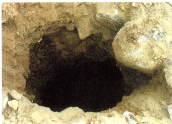
This collapse only became apparent when the topsoil was removed (Donal Daly)
